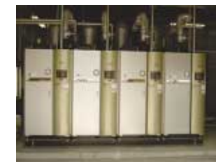
Natural gas boilers
